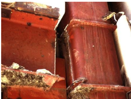
c) Damage from Kobe earthquake
